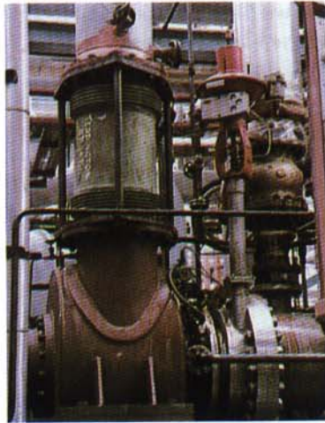
A petrochemical plant using a multi-tied expansion joint to absorb pipework deflections and minimize stresses.
