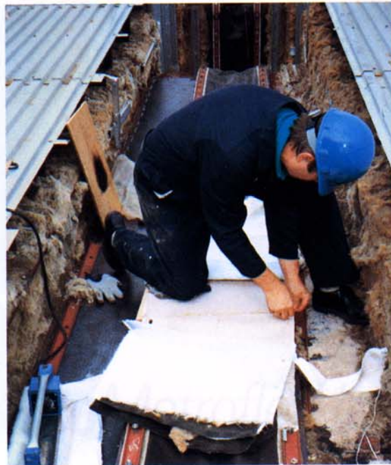
A WahlcoMetroflex technician prepares to hot splice an expansion joint. An overview of the splicing procedure is shown on page 9.
